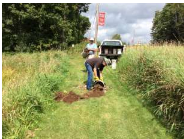
A deep hole suddenly developed in the grassy path leading into the Wetland Park. Volunteers Norbert, Darlene, and Tom filled it with 30 buckets of stone and dirt and will monitor its condition in the future.
